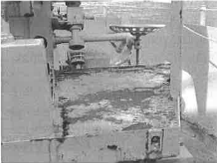
One of three platforms we repaired. This one is at the trainer's platform and was the worst one.
