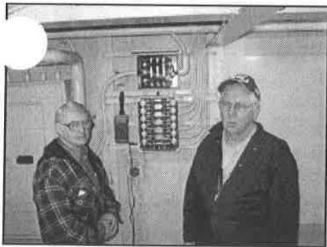
Jack Floyd and Lee Mowan in the process of checking out the fuse panel in our exhibit area.
