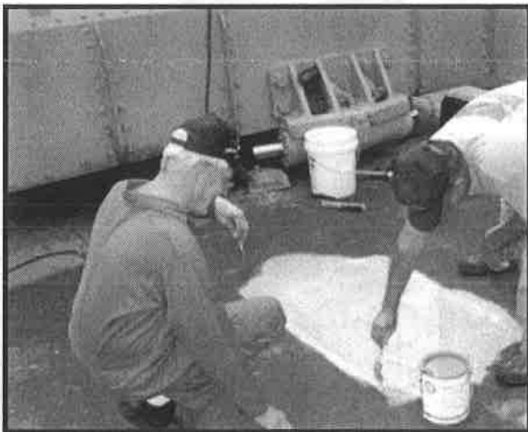
Jim and Roland putting a coat of primer on new section of deck.
