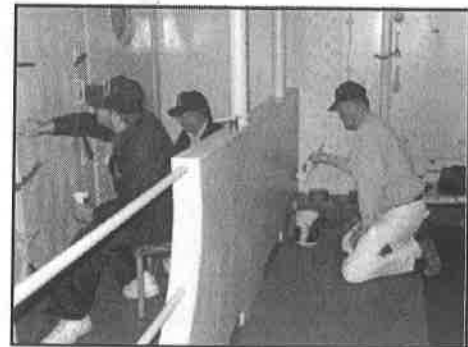
Tom Giardina, Don Batty and Roland Cote painting exterior of radar room.
